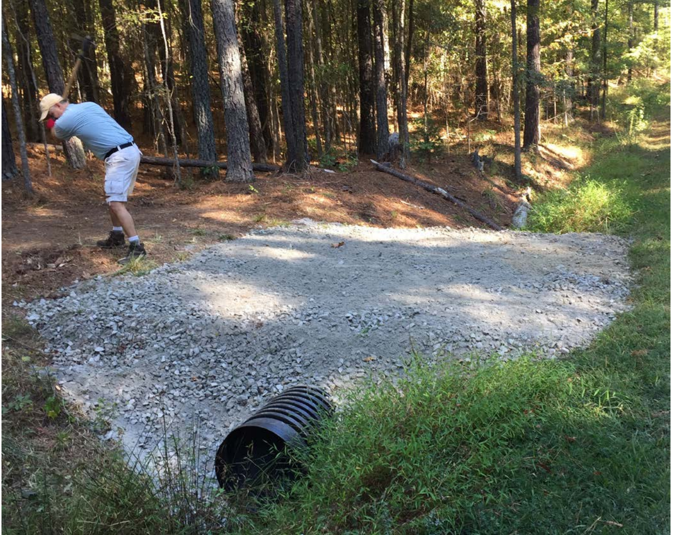
Finishing up work on covering culvert for new connector at Pittard Sears
